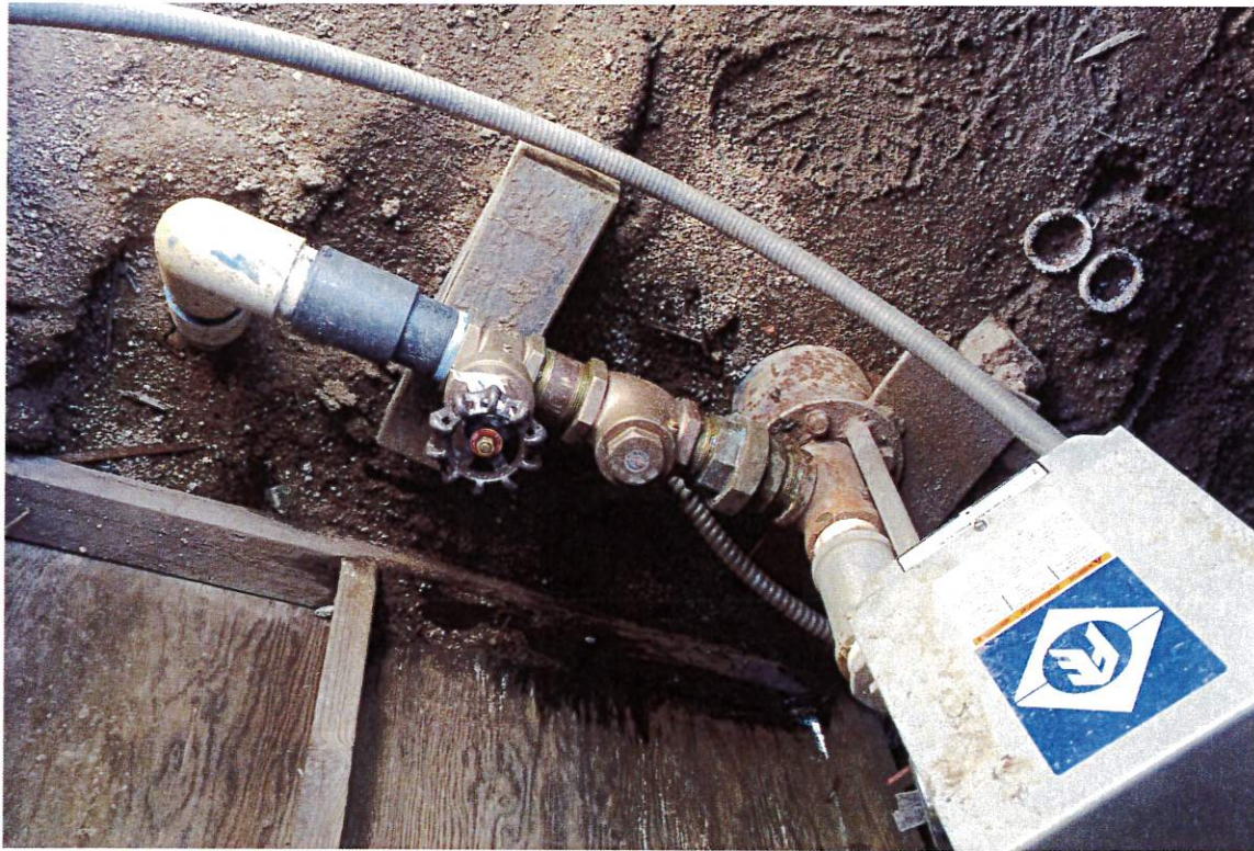
well # 1 New gate valve.
