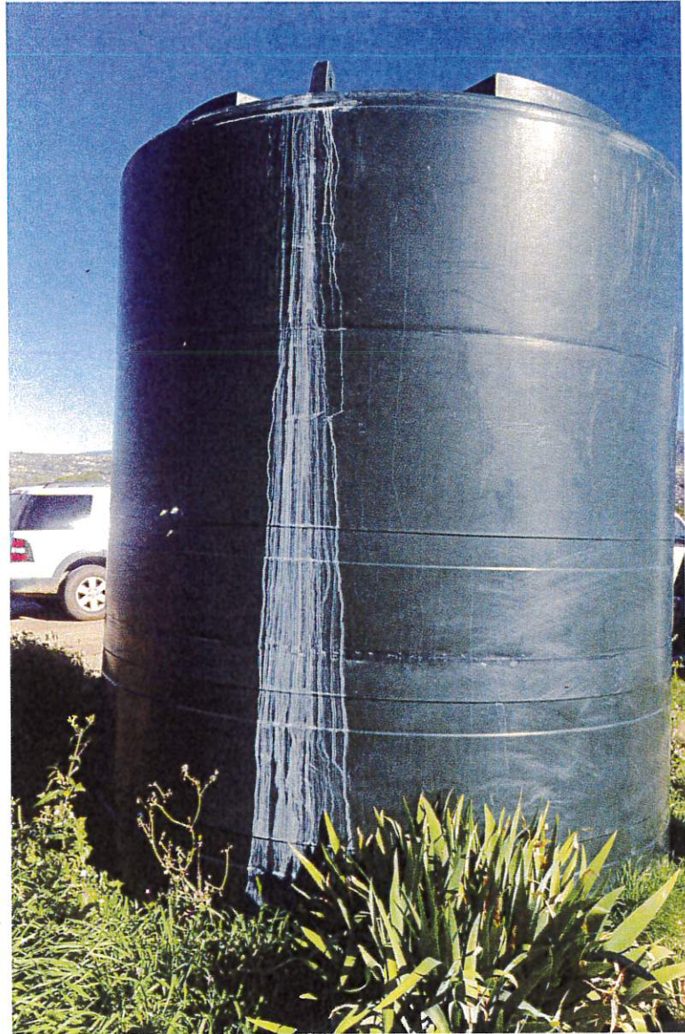
Reservoir Top of Mill Float's inoperative. Needs repair
